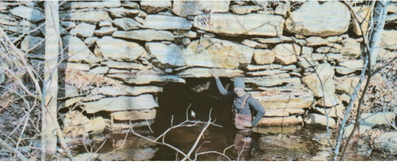
Photo courtesy of Tighe & Bond Jonathan Ives, a senior project manager at Tighe & Bond, inspects damage to the bridge on Sport Hill Road that was caused by last August’s storm.
